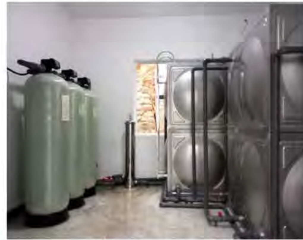
Water works Rural Drinking Water
